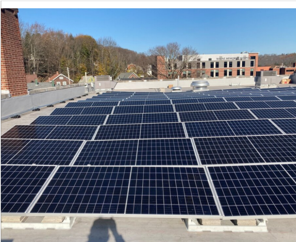
The Stourbridge Project solar array in place, looking north toward Wayne Memorial Hospital in the background.
